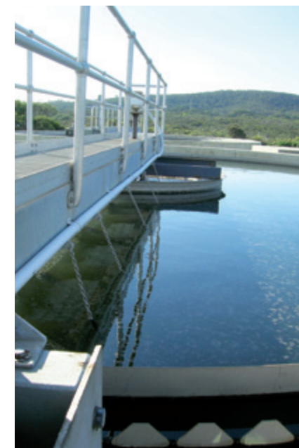
Fig. 4.5: Final sedimentation tank in a conventional waste water treatment plant (© ISA, RWTH Aachen)
